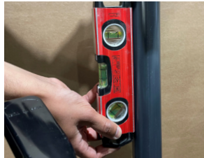
Check blower is vertical
